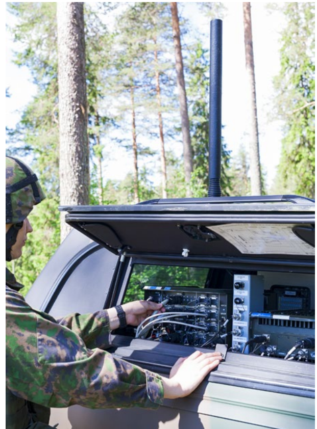
Figure 6: Bittium TAC WIN installation in an FDF Army signal vehicle.
